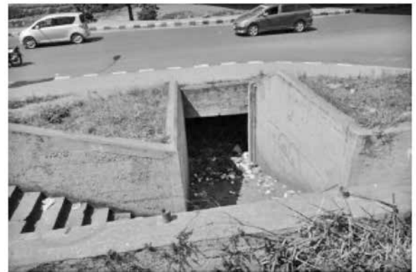
FIGURE 5 Dark and unkempt underground walkways Source: Authors 2017
